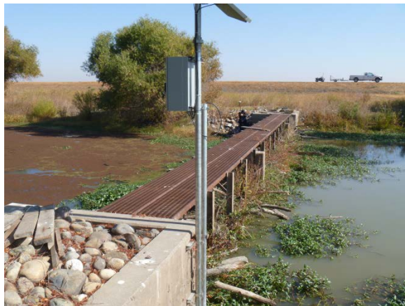
Photo D-4 Lower Merced Weir Showing Debris Accumulation Upstream of Weir
