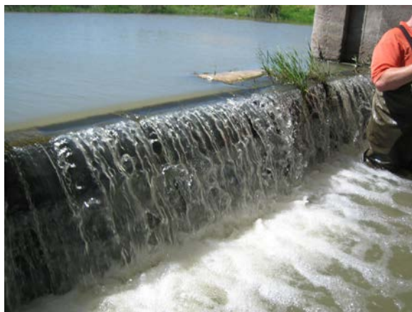
Photo B-3 Boards Located at the Structure Inlet at the Radial Gate Seal
