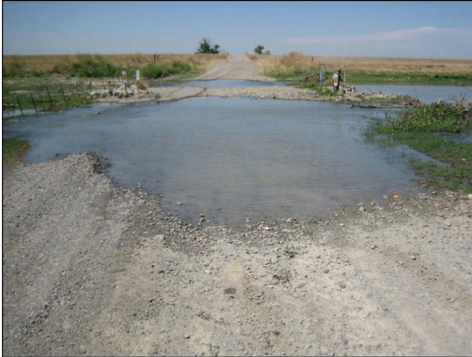
Photo 2 Dan McNamara Road when Partially Overtopped
