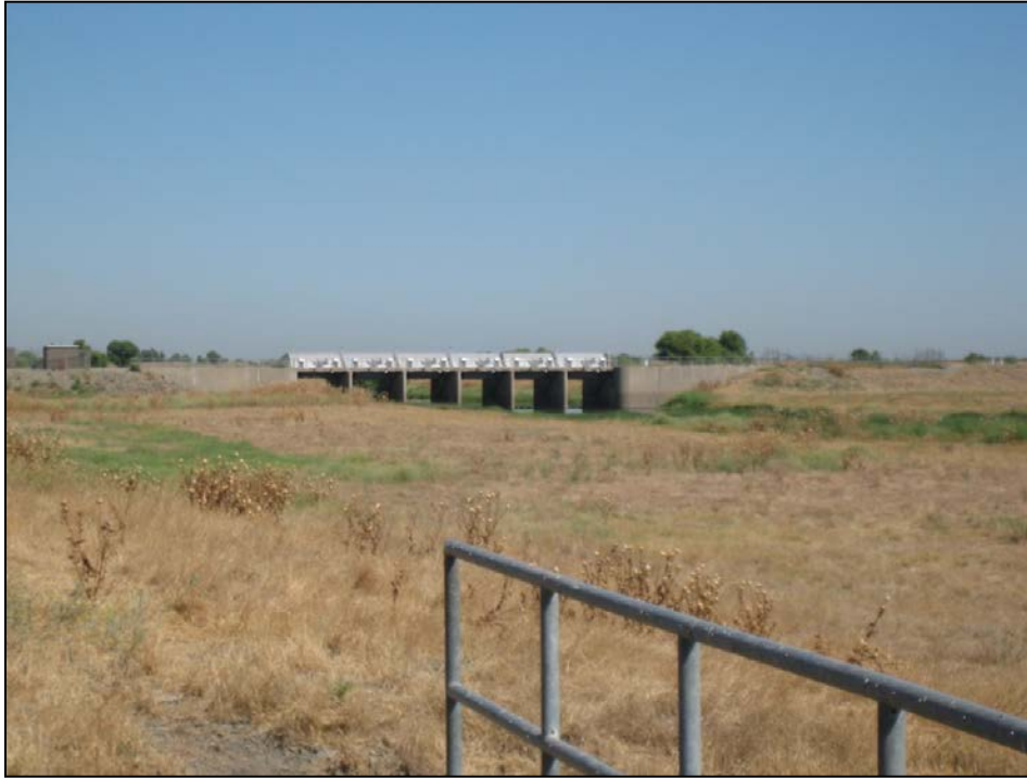
Photo 1 Eastside Bypass Control Structure from the Mariposa Bypass Control Structure Looking Downstream at the Eastside Bypass
