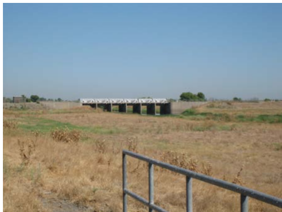
Photo B-1 Eastside Bypass Control Structure from the Mariposa Bypass Control Structure looking Downstream in the Eastside Bypass
