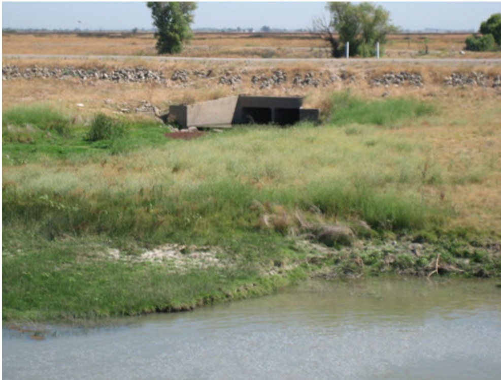
Photo B-5 Owens Creek Overflow Structure Downstream the EBCS on the Right Bank
