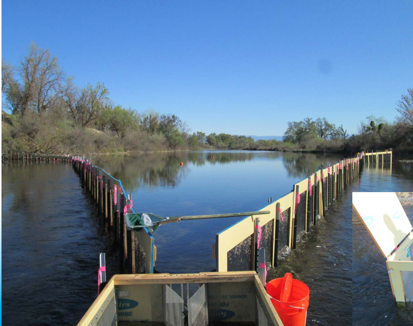
Weir collection box
