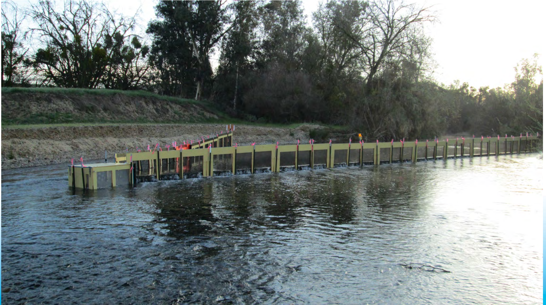
Fish Collection Weir at Scout Island
