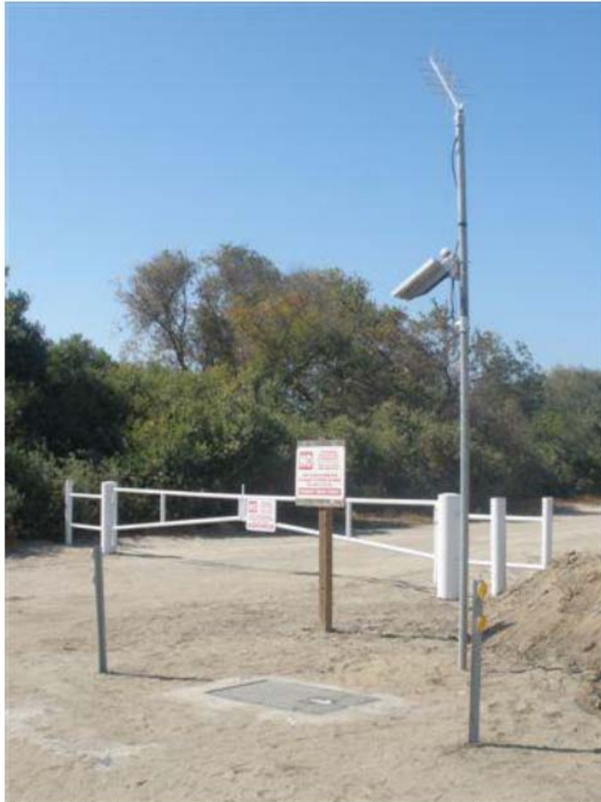
Well and data logger are below-ground in a vault (foreground). Power is supplied by a solar panel on the pole, and data are transmitted via satellite using the antenna on top of the pole.
