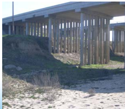
Degradation in Eastside Bypass
