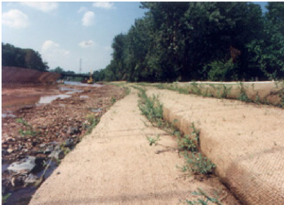
Figure 5-18.—Example installation of FES showing layers of FES with willows planted between layers.
