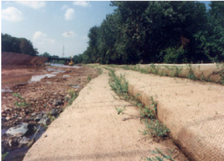
Figure 4-9.—Example installation of FES showing layers of FES with willows planted between layers.
