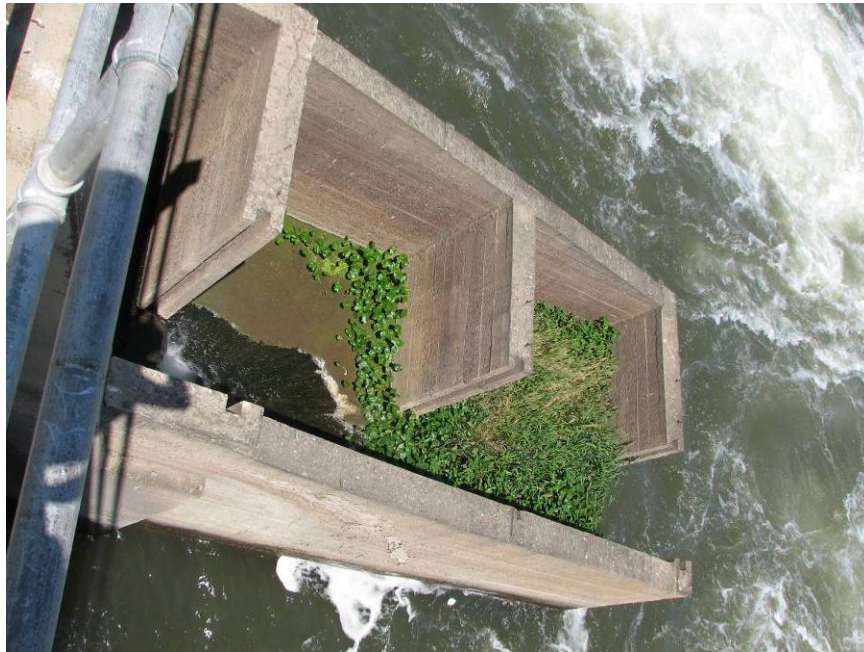
Figure 2-1 Mendota Dam fish ladder
