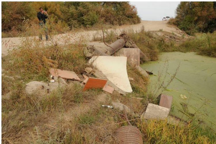
Figure 1-10 San Mateo Avenue crossing of Reach 2B showing single culvert beneath the road
