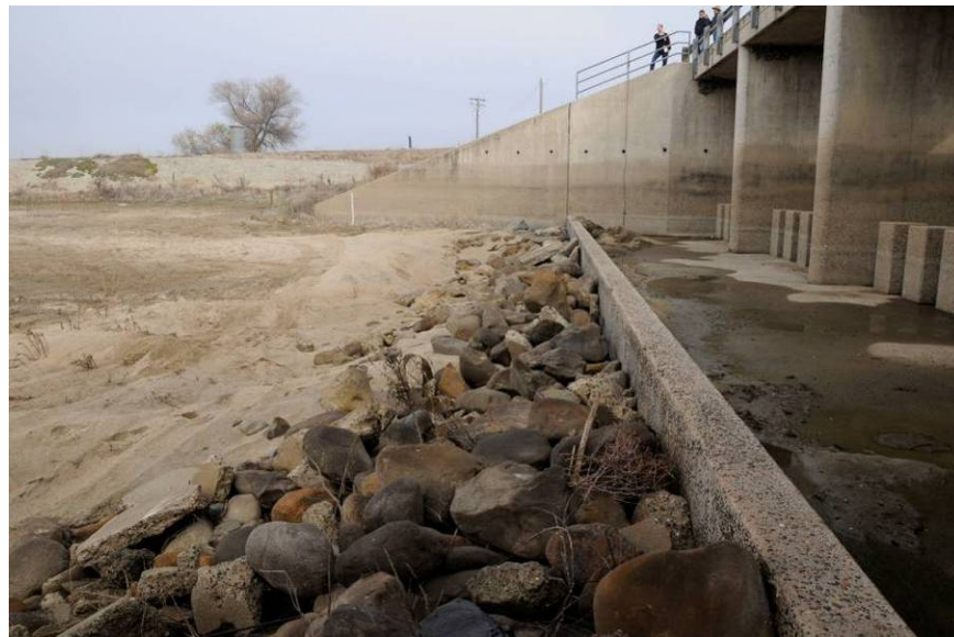
Figure 1-8 The concrete weir and bordering rip rap along the downstream edge of the Chowchilla Bifurcation Structure in Reach 2B
