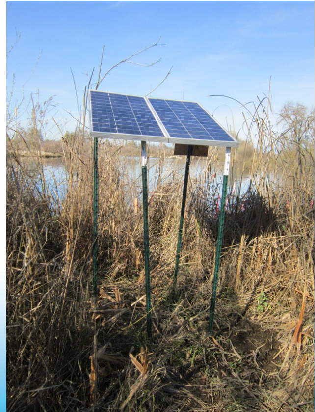
Solar panels to charge batteries
