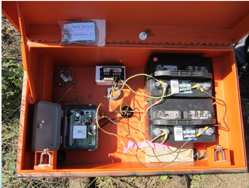
Lockbox with receiver and batteries
