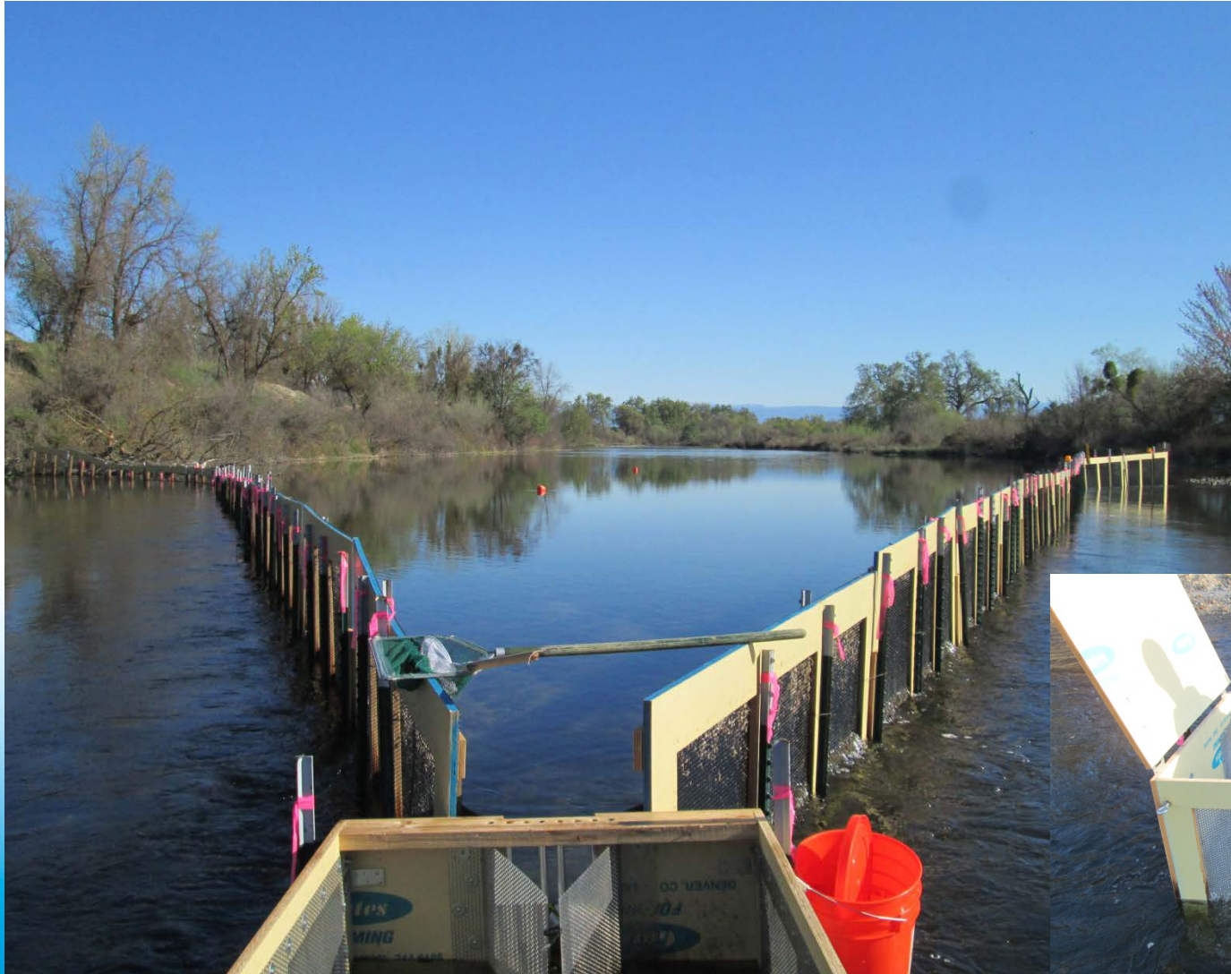
Weir Collection Box
