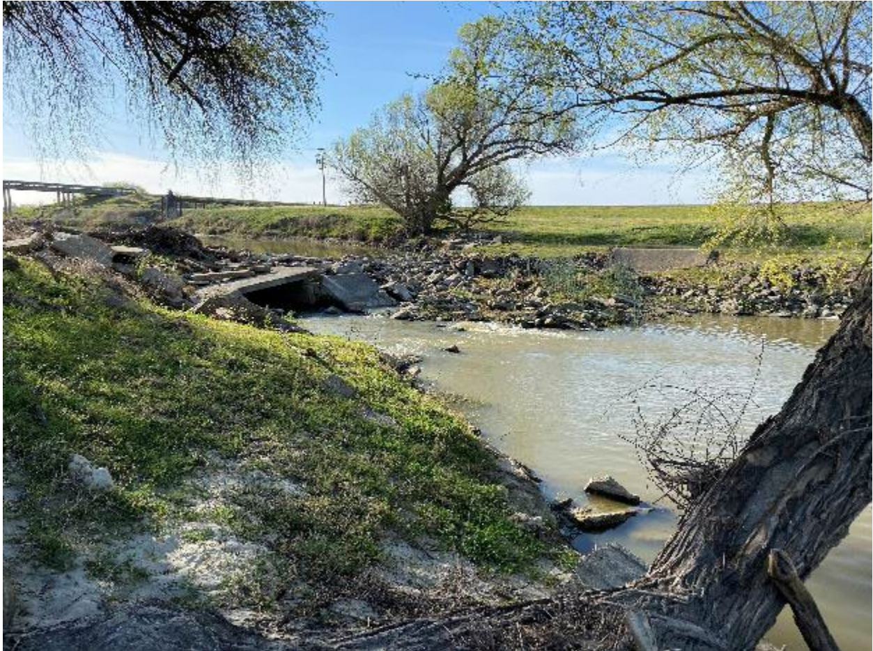
Figure A-1. — Image of Eastside Bypass Rock Weir during 2021 spring-run Chinook Salmon ( Oncorhynchus tshawytscha ) adult trap and haul and monitoring efforts. During 2021 monitoring, this location was deemed the first impediment to upstream passage of adult salmonids and no sampling was completed upstream of this location.
