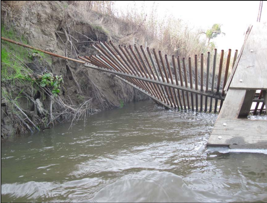
Figure 13.—Bank erosion and scoring causes holes in the barrier which may provide upstream passage at the Hills Ferry Barrier.
