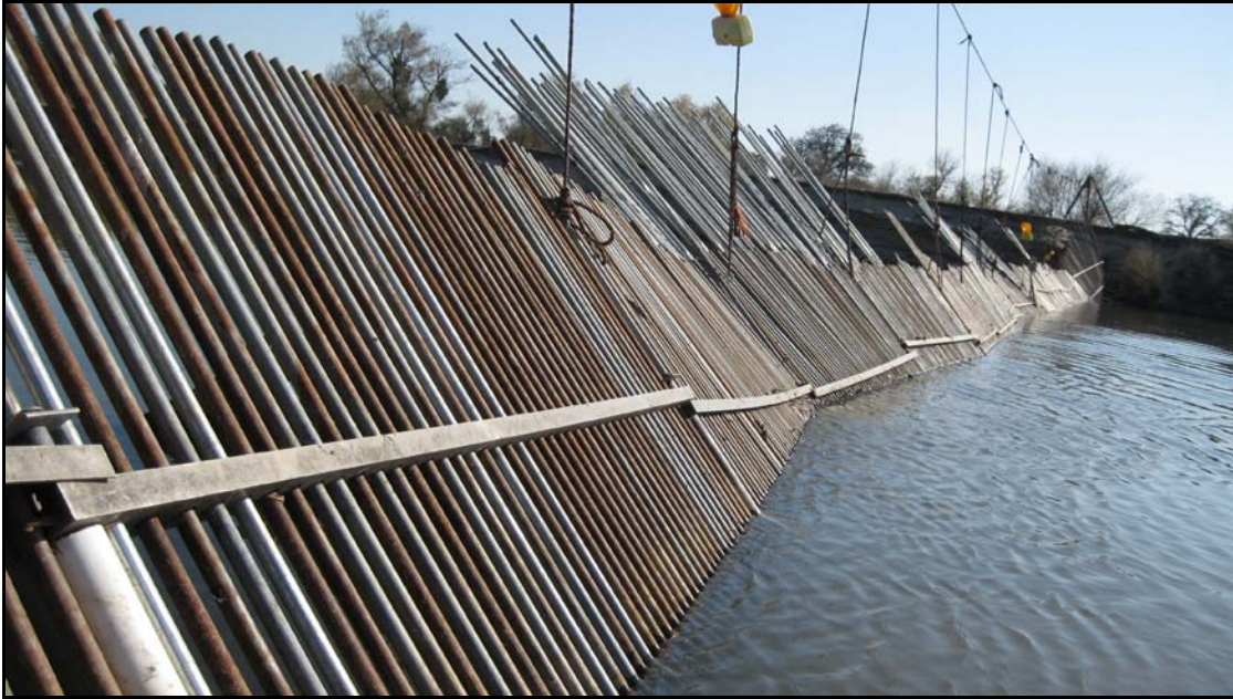
Figure 3.—Hills Ferry Barrier is a sliding pipe weir constructed of aluminum channel with 2.5-cm (1-in) holes that allow 1.9-cm (.75-in) electrical conduit to slide freely vertically in the corresponding holes and are pushed into the riverbed.
