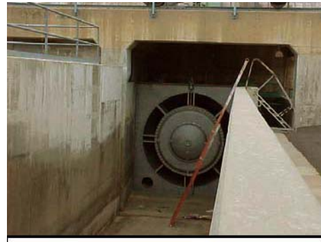
Frontal View of Madera Canal Outlet Works at Friant Dam
