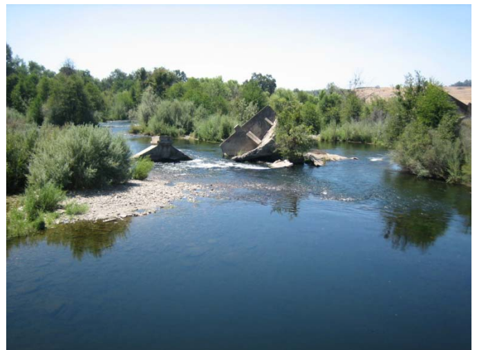
Photo 2_B. Bridge debris from Road 206 Bridge looking downstream
