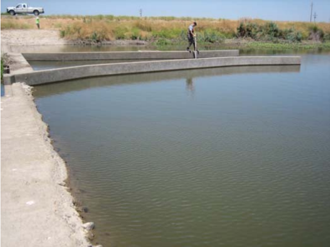
Photo 29_C. Sand Slough Control Structure flume from right bank
