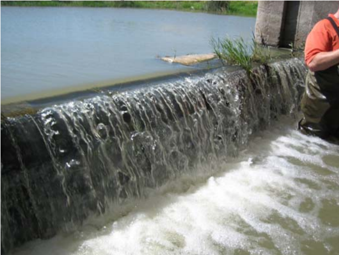
Photo 48_C. Weir upstream radial gate seal
