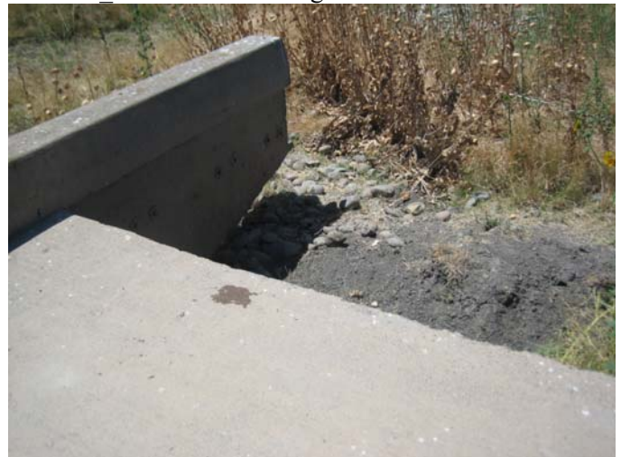
Photo 50_B. Erosion of bridge on left bank
