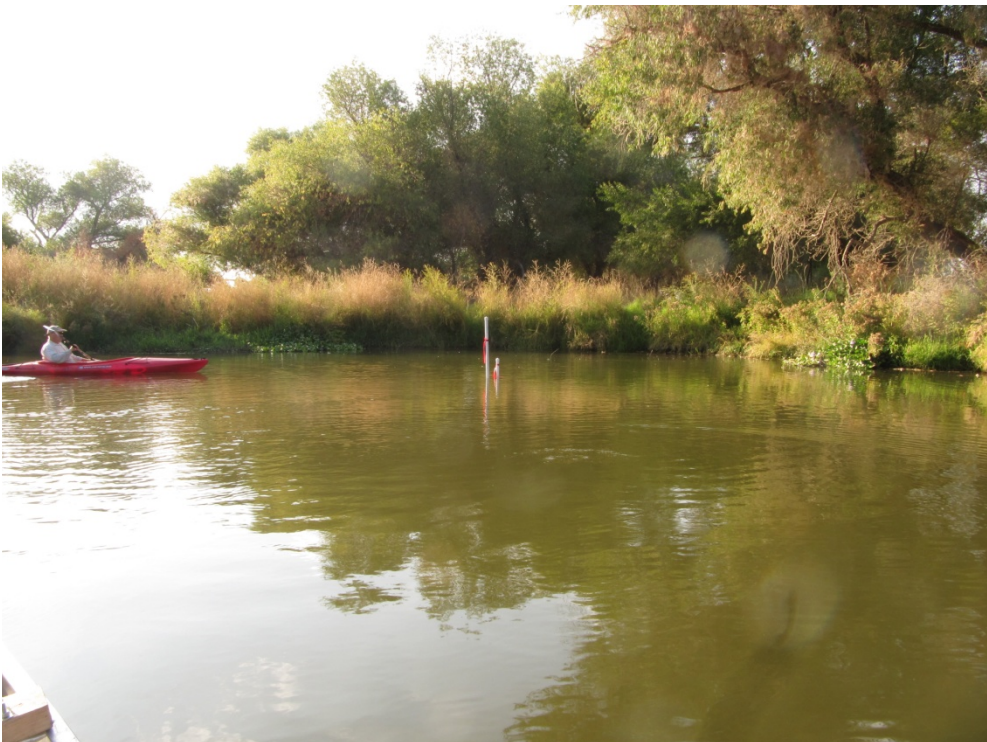
Figure A-4: View of sensor array installation in SJR 193.24(2) looking downstream.
