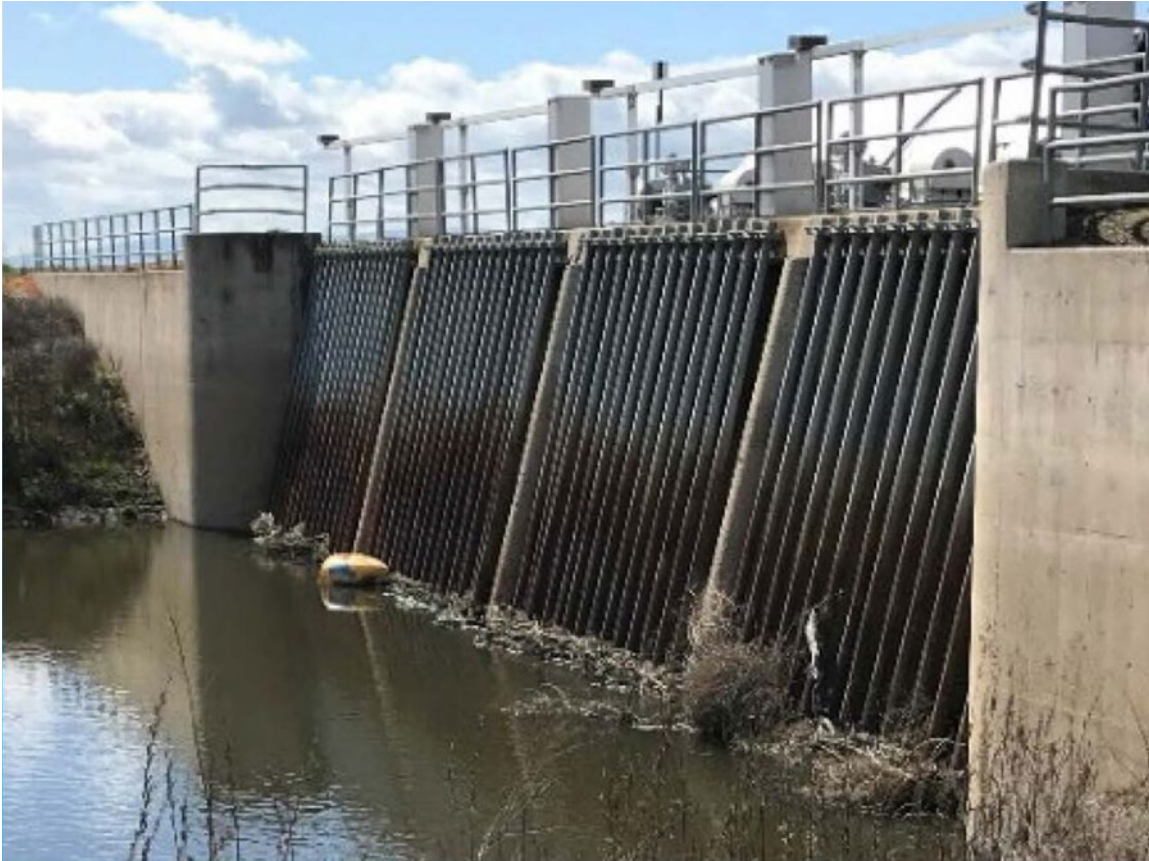
Figure 3. Image of the trash rack on the upstream side of the San Joaquin Bifurcation Structure. Photo courtesy of Department of Water Resources.
