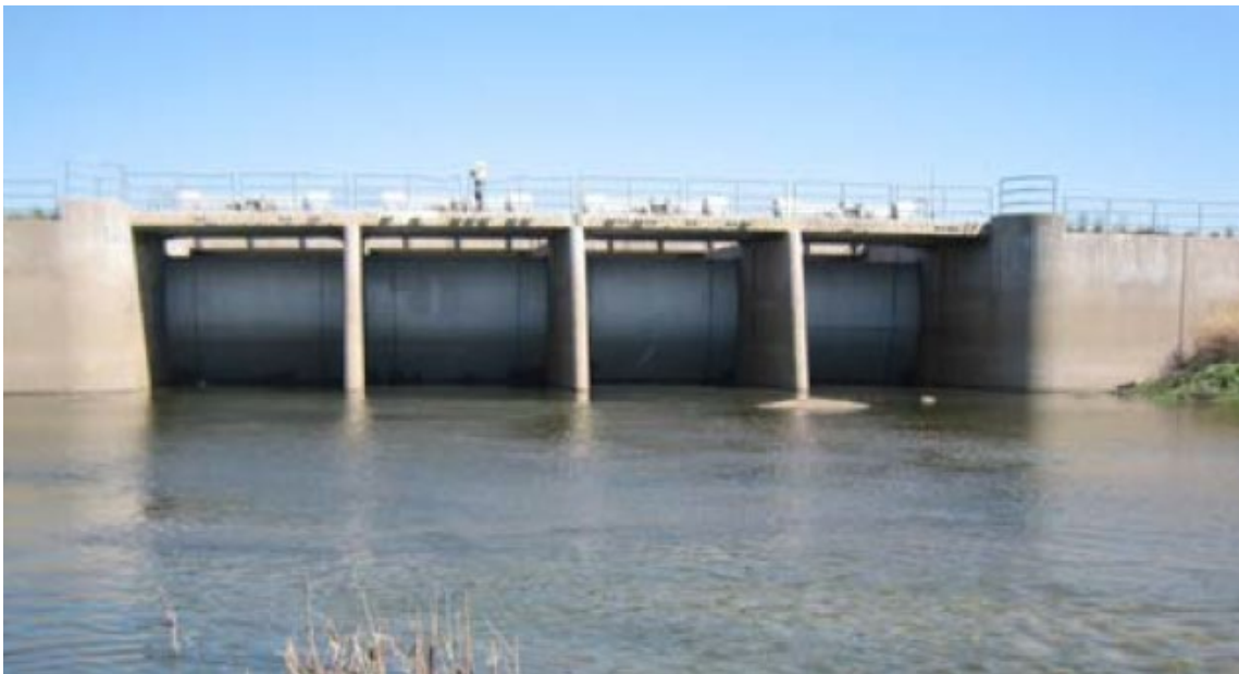
Figure 2. Photo looking downstream at the Chowchilla Bifurcation Structure radial gates leading into the Chowchilla Bypass. Photo courtesy of Department of Water Resources.
