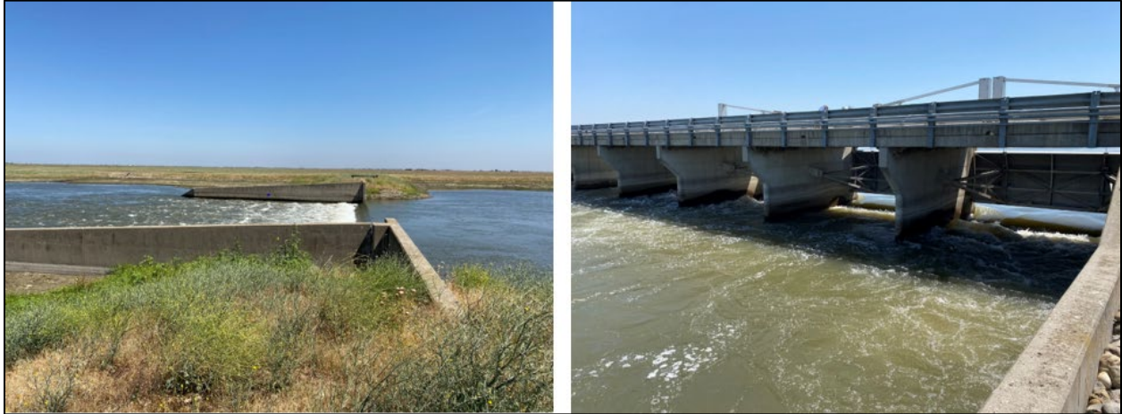
Figure 5 Mariposa Bypass Structures. (Left) Drop structure at the downstream end. (Right) Control structure at the upstream end.
