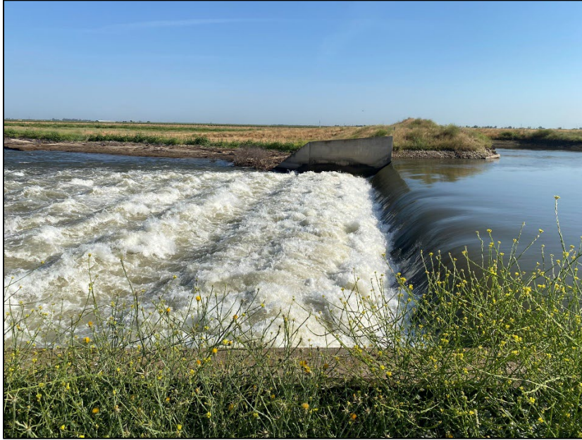
Figure 2 Drop 2 structure with high velocities and a drop that can prevent fish passage upstream
