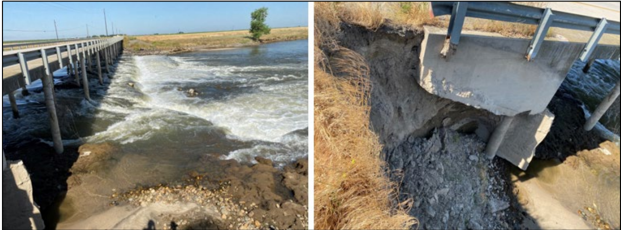
Figure 3 Avenue 18.5 Bridge. (Left) Observed drop downstream of the bridge with high velocities from the right bank. (Right) Eroded right approach embankment exposing the abutment.
